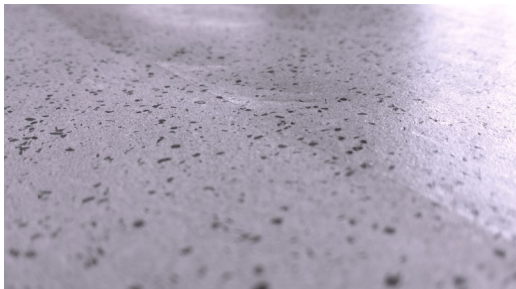
Left at the bottom: unprotected
